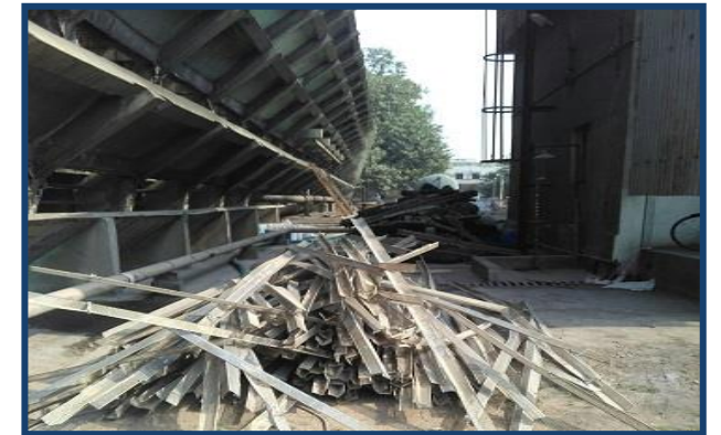
V Bars & drift eliminators in CT
