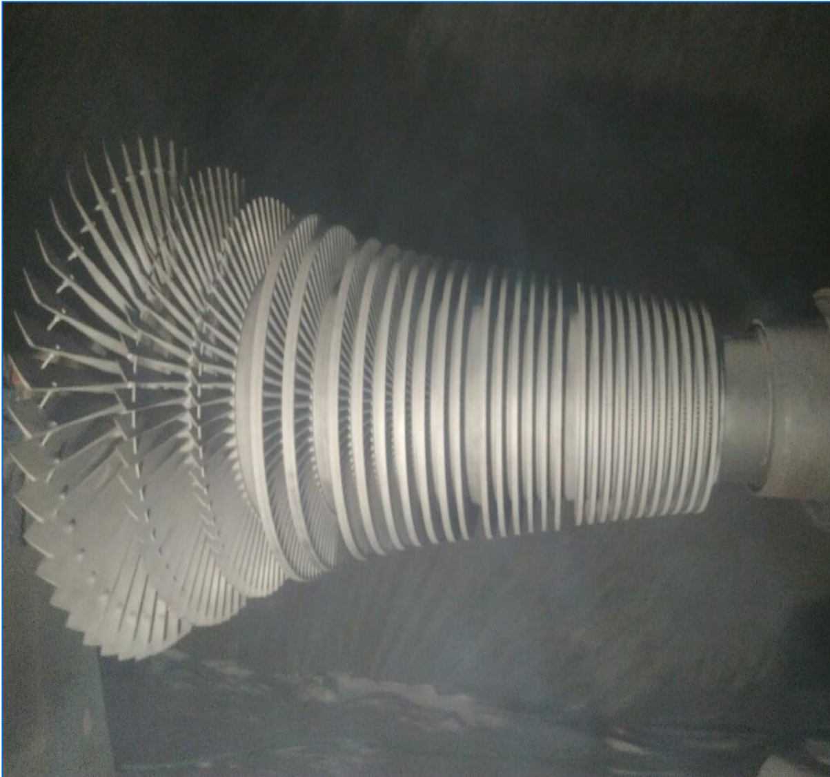
Unit-1 Existing 67.5 MW Turbine Rotor
